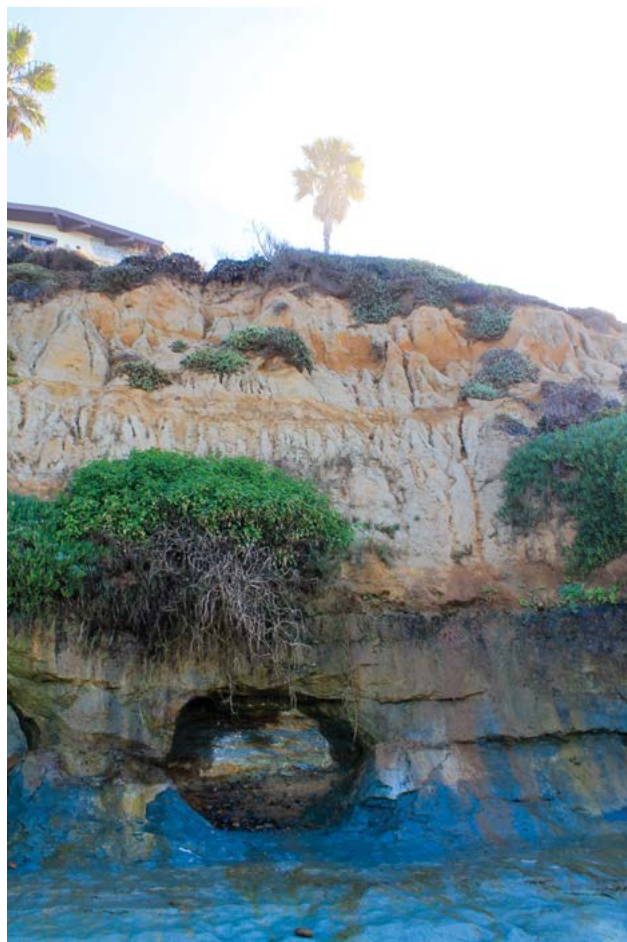
Southern California's oceanside cliffs are fissure-prone. Sun and wind erode them while water tapers their faces into rills and seeps into their presumed solidity.
