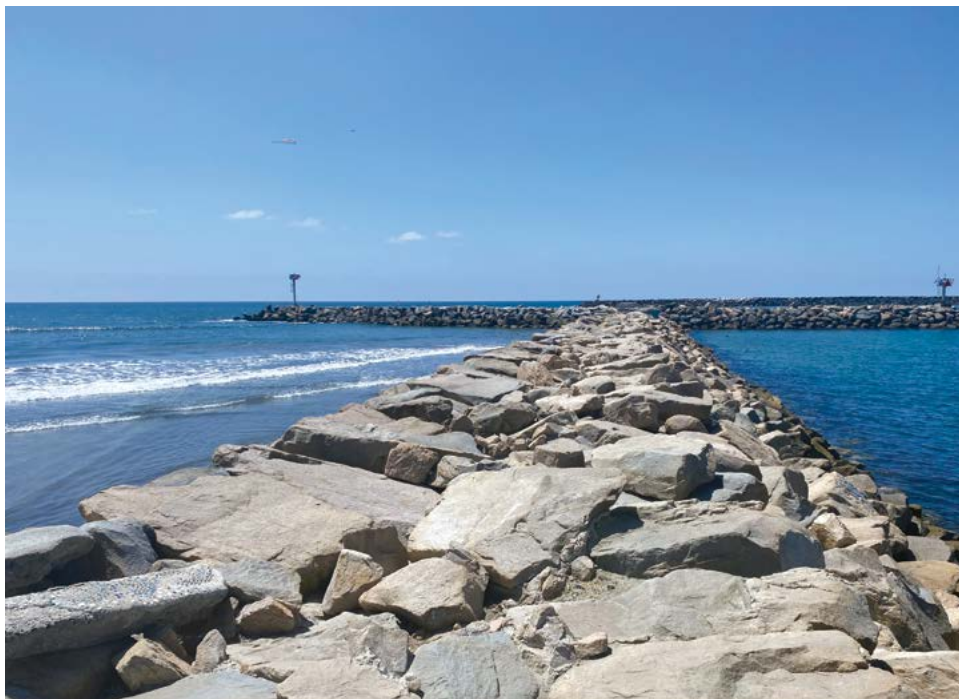
The large jetty that protects the two harbors in Oceanside, which share an entrance to the ocean, creates a barrier that blocks the sand that would naturally be carried south by ocean currents.
