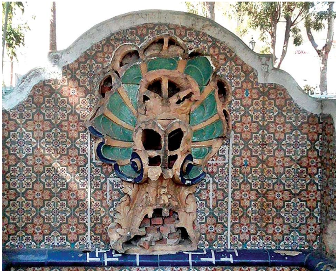
The vandalized faun before restoration.
