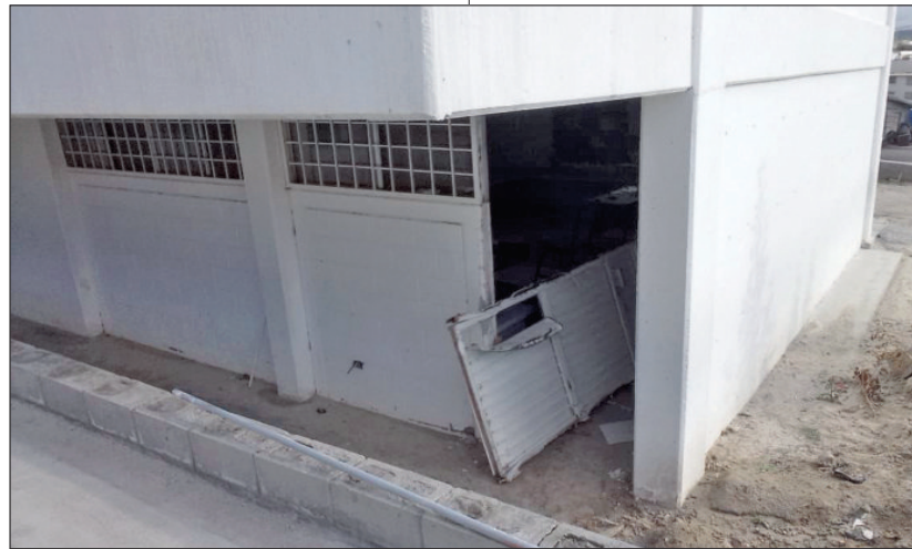
Principal Cristian Gastelum calculates that 60 percent of the school infrastructure was stolen or vandalized.
