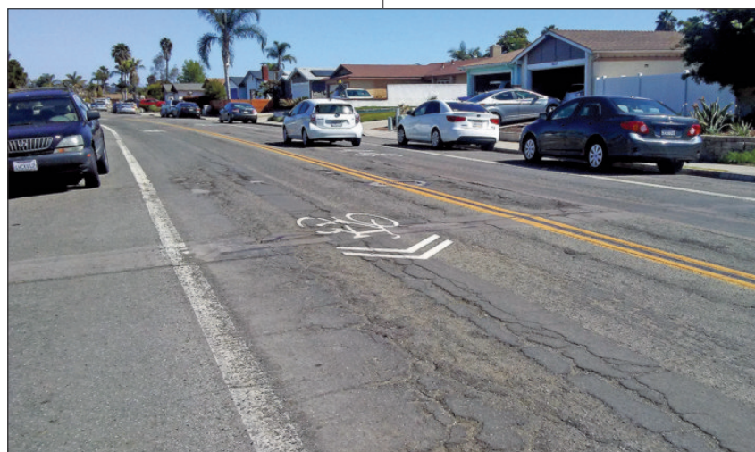
Gold Coast Drive. "The road's failure is not from normal wear and tear. Its badly built subsurface finally deteriorated so badly it can't be fixed."
