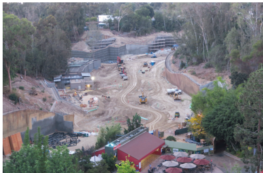
Construction shot of Africa Rocks in 2016, which would open a year later in what used to be Dog and Cat Canyon.
