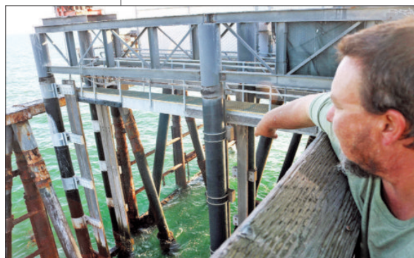
Nick Cline- “They have all of this excellent foundation underneath the old boat launch area.”
