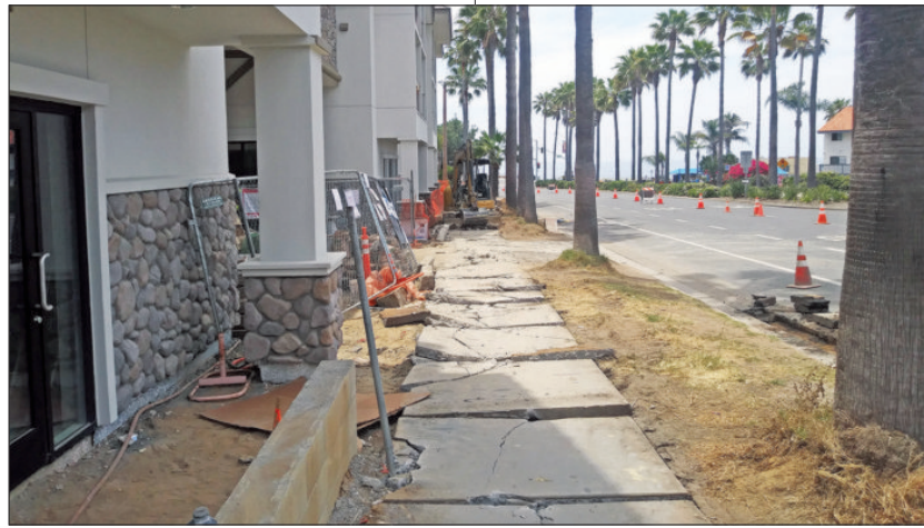
SpringHill Suites has emerged from the winter of its discontent and is back under construction.
