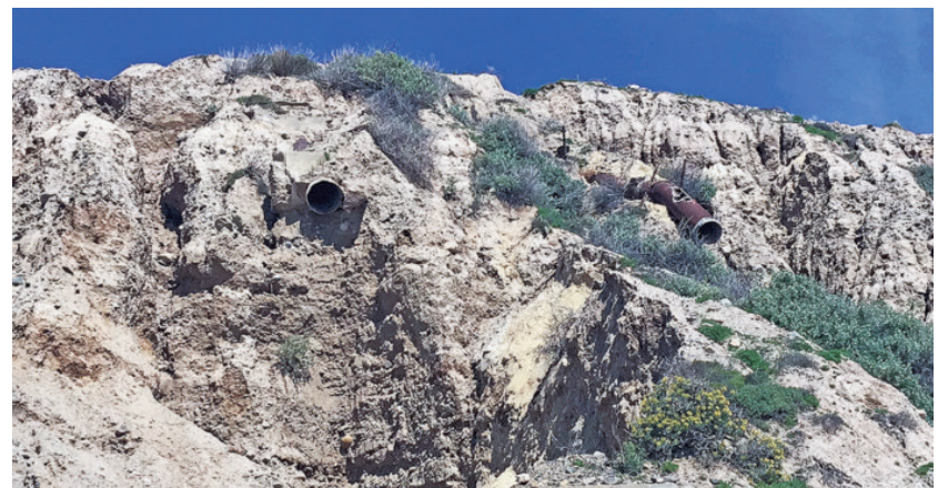
Outfalls: attempts to steer water away from cliffs don't prevent erosion.
