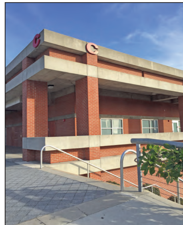
Millions were spent renovating the C building at City College. But wiring crucial to the Radio, TV and Film department was not functional upon completion.
