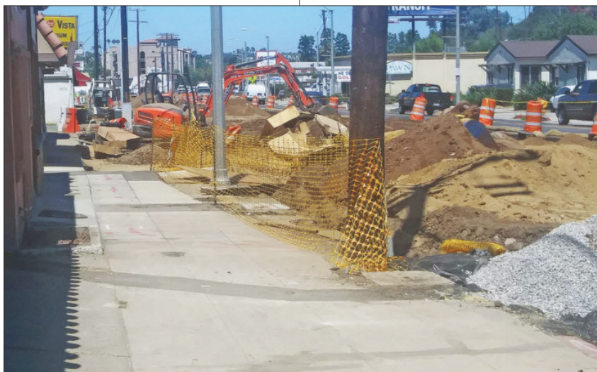
“They don’t even clean up their work. They leave piles of asphalt on the sidewalk.”
