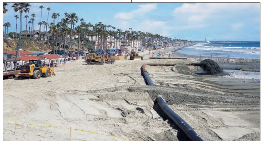
Pumping dredged silt and sand from the Oceanside Harbor to Tyson Street beach.
