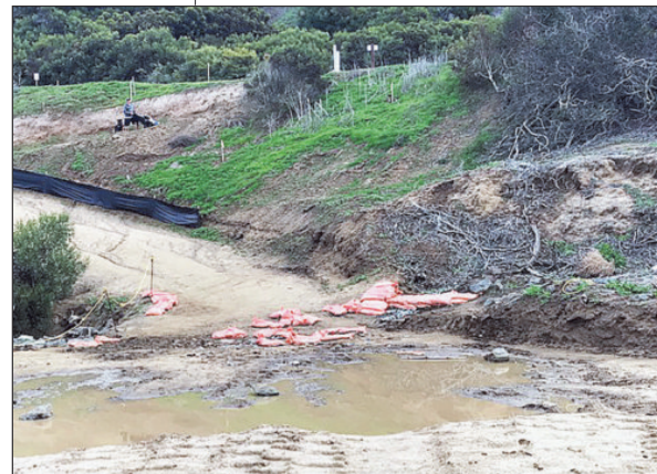
Recent rains have washed away vegetation and pathways.
