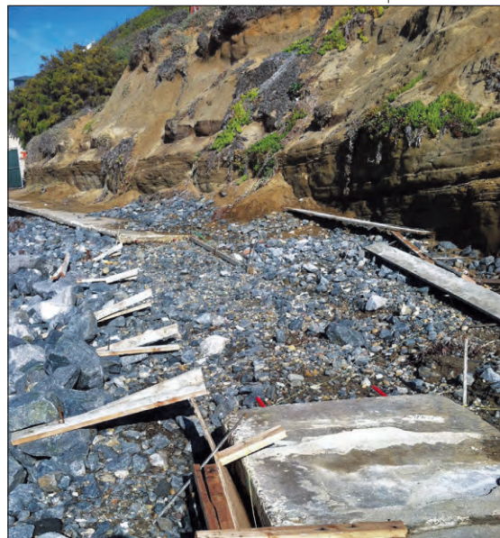
Orchard repairs washed away.
