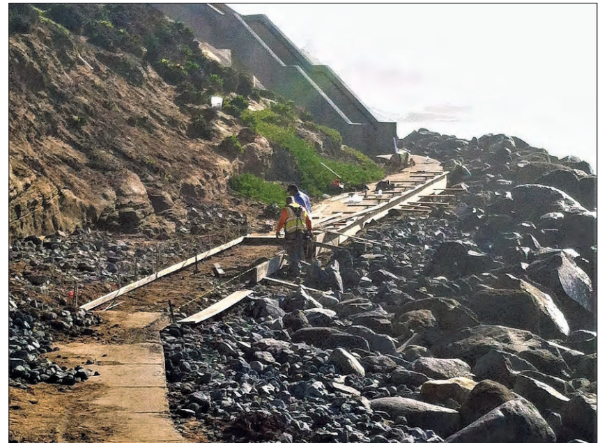
Photo of work in progress on December 17 at Orchard Ave improvement project. Stabilizing the gutted sidewalk. Looks like they're forming for concrete.
