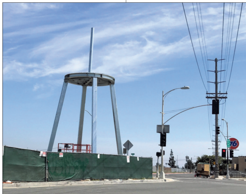
For now, the “water tower” looks more like a tripod from War of the Worlds
