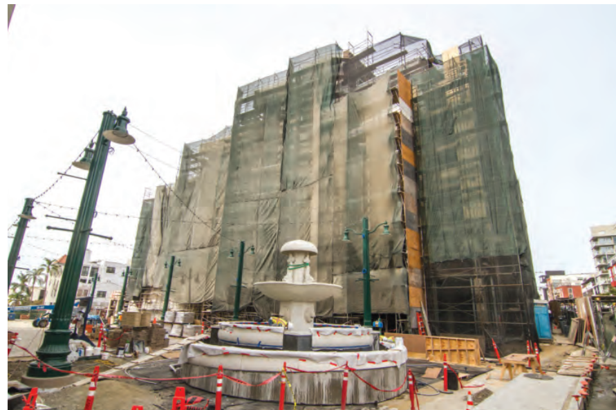
Piazza della Famiglia is being constructed on the section of Date Street between Columbia and India Streets. The condo tower in the background is on the former site of the Reader building.
